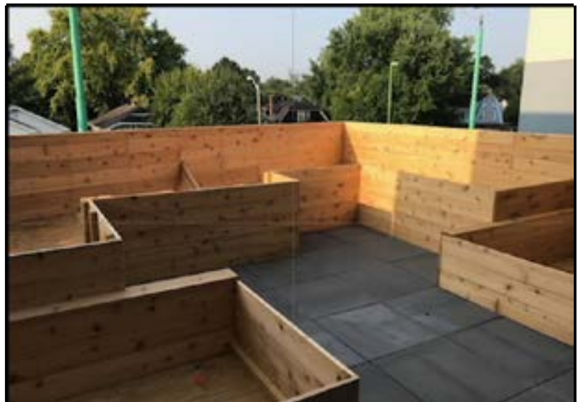
New rooftop deck with multiple planter-bed availability at Paramount School of Excellence
